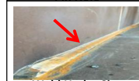
Weld Under Size
